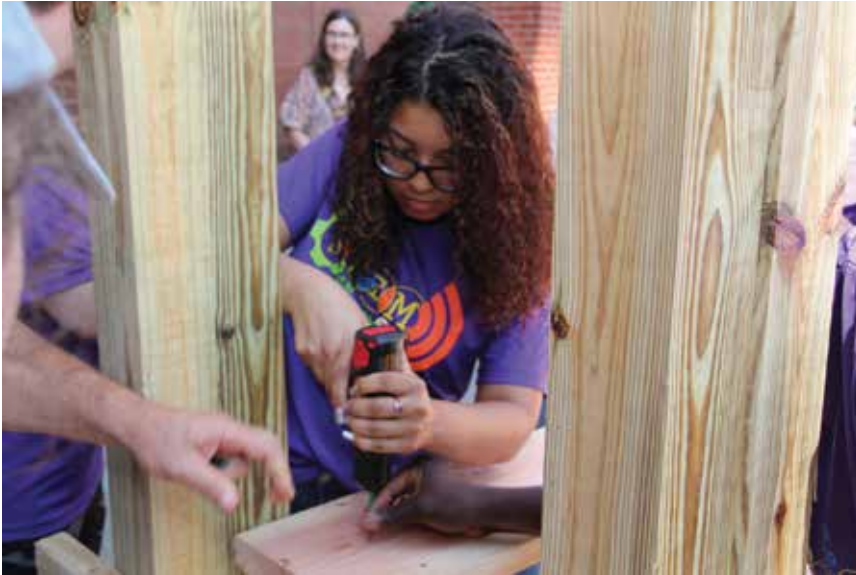
Student helps build a working demonstration bridge during STEM Starter Academy's annual Summer Bridge Program.
