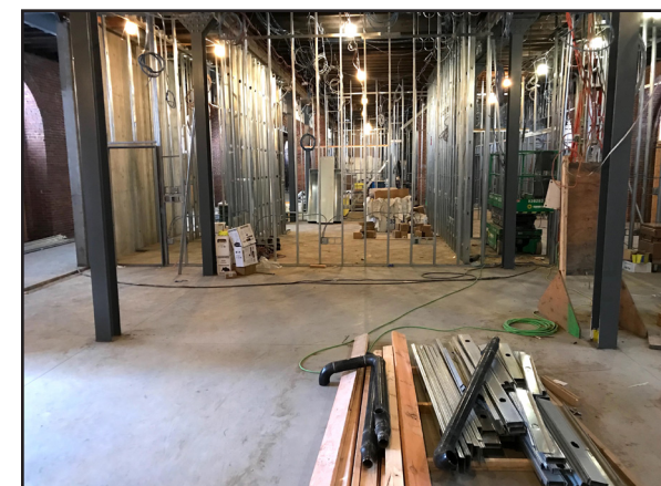
Emerging from the west end of the eating commons, one will encounter various offices including that for Student Activities. The skeletal metal superstructures outline future office dimensions. USB connectors and chargers will be situated throughout this massive, state of the art facility.
